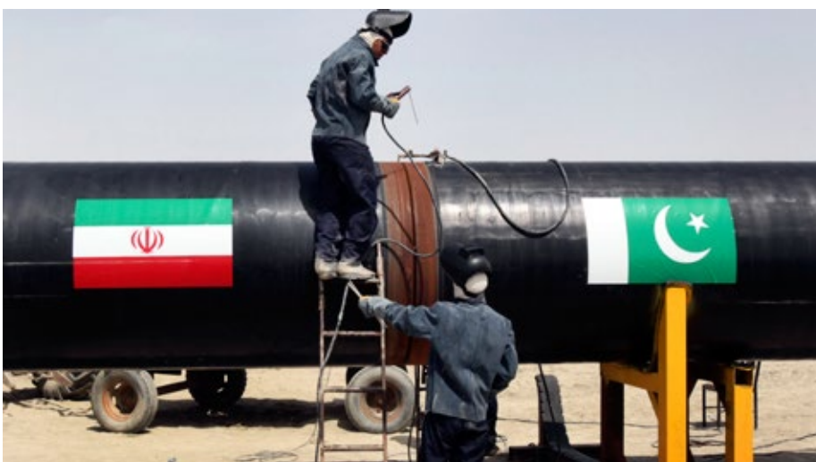
Iranian workers weld a joint on the Iran-Pakistan pipeline. It could provide 21.2 MMcm/d by 2020. (PA)
