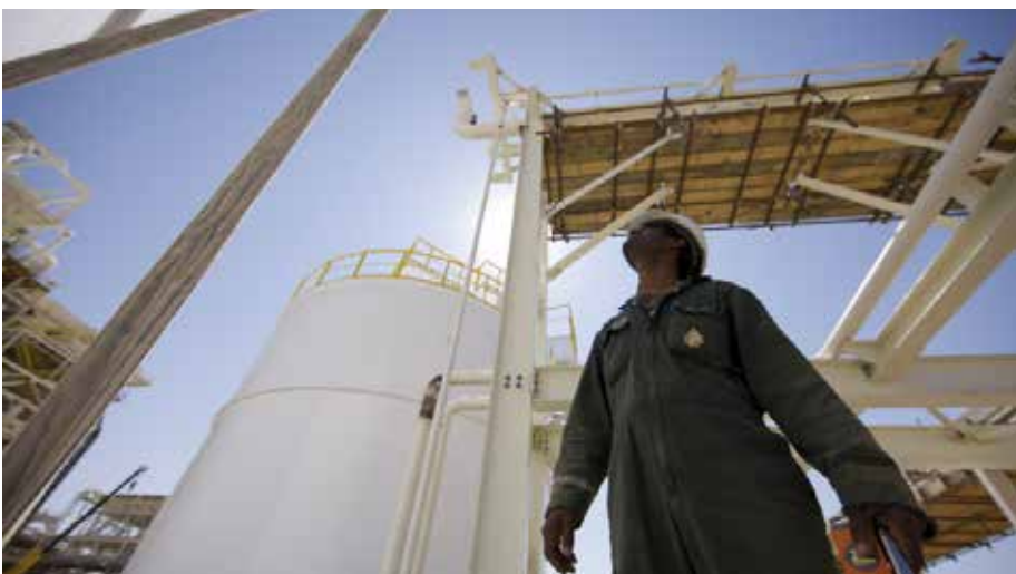
A Shell gas storage tank in Oman, where the company employs enhanced oil recovery techniques. (Shell)
